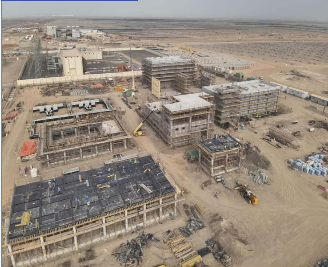
Manah Substation for Manah I & II Solar IPPs
